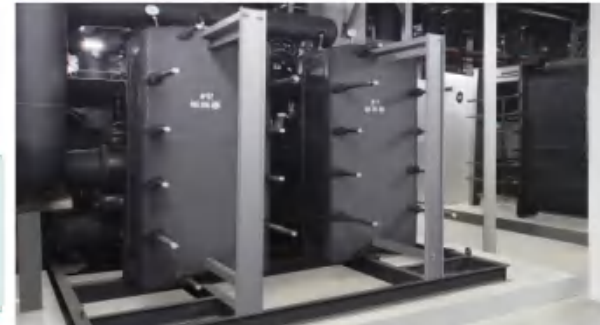
National Supercomputer Center in Guangzhou (Tianhe-2), Guangzhou, Guangdong
