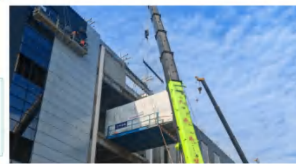
XX Cloud Data Center, Wuhu, Anhui
