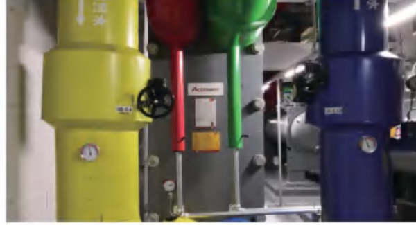
Beijing City Cloud Data Center, Beijing
