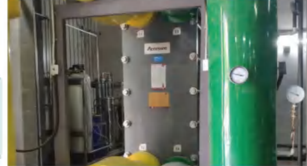
State Grid Intelligent IoT Data Center, Beijing
