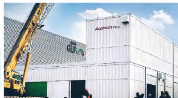
GLP Changshu Southeast Data Center, Jiangsu
