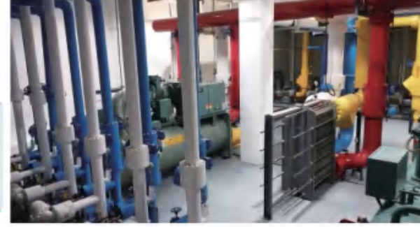
China Telecom Cloud Computing Base, Qingdao, Shandong
