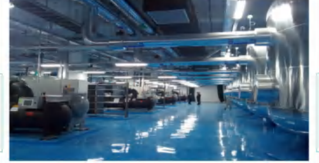
Huawei Cloud Data Center, Daqing, Heilongjiang
