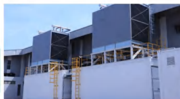
XX Data Center, Penang, Malaysia
