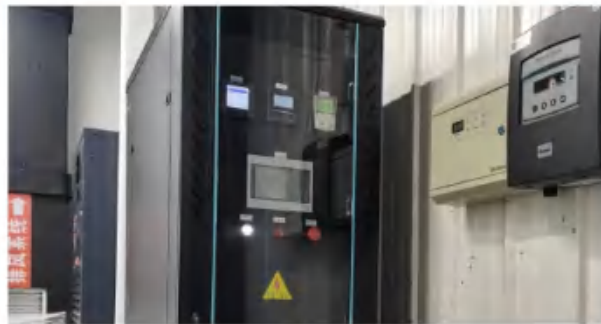
GLP Liquid Cooling Pilot Project, Changshu, Jiangsu
